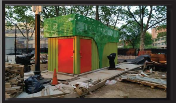
Refurbished Sea Container Brooklyn, NYC
